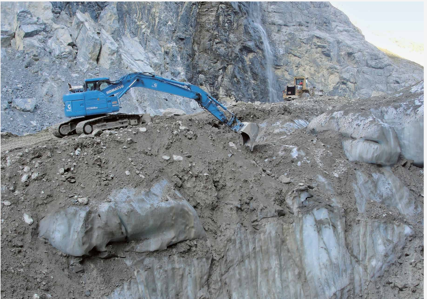
Construction work on the Unterer Grindelwald Glacier (Canton Bern) on 7 October 2009: The glacier has retreated to a huge extent in the last 150 years. In 2005 a lake formed for the first time on its surface. In 2009 a drainage tunnel was built in order to avert the danger of a glacial lake outburst flood.
